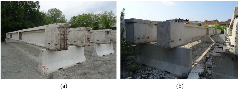
Figure 1. Views of PC bridge deck beams in the testing site: (a) Detail of a group of beams; (b) PC beam with (left) and without (right) top slab.
