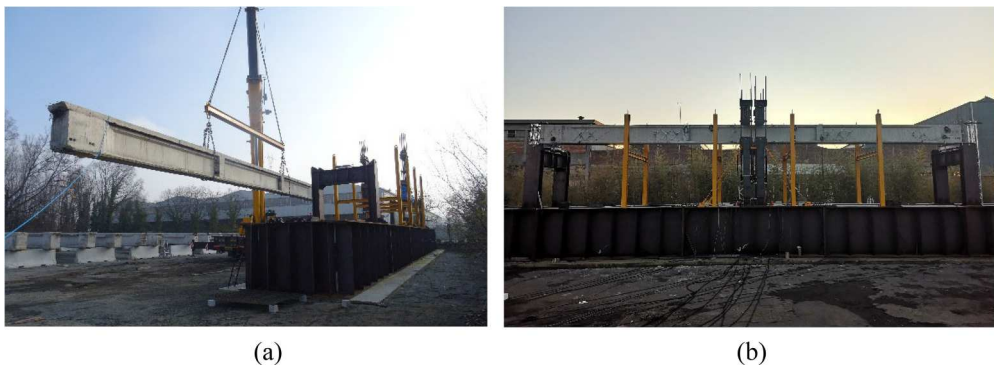
Figure 12. Full-scale load tests: (a) Lifting of a beam over the testing frame; (b) View of the testing framework with the PC deck beam without RC slab during the test.
