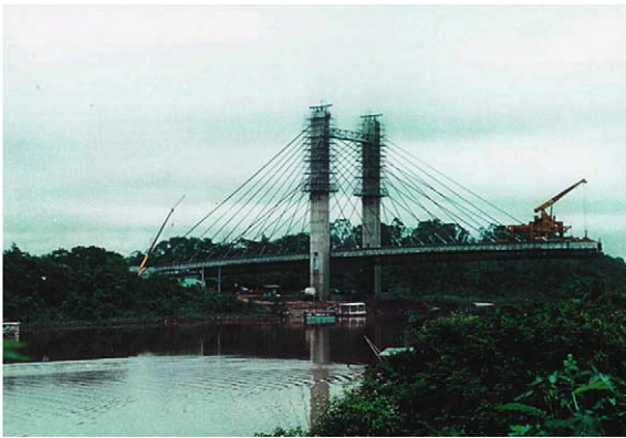
Fig. 15. Cable-stayed bridge over Cujaba River in Brazil. Two photographic views of the bridge during construction.
